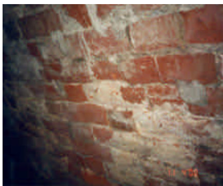
Figure 3 Efflorescence and crypto-efflorescence damages on the vault ceiling
