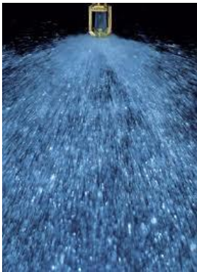
(a) Water deluge system
