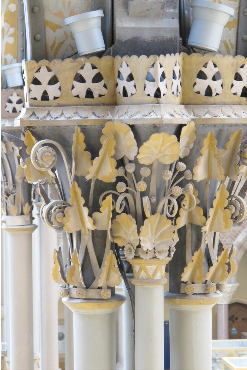
Figure 3 Cast-iron columns with wrought-iron capital, imitating botanical forms. Courtesy of the Oxford University Museum of Natural History. Photograph by author, 2015.
