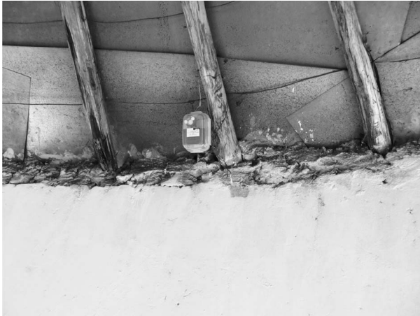
Figure 2 Carbon dioxide sensor mounted in the rafters of the church at approximately 2 m height.
