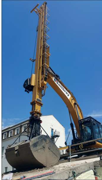
Figure 7. The innovation programme led to use of telescopic clamshell excavators on other projects following successful trials at Paddington, which found excavation rates increased from 48 m 3 /h to 54 m 3 /h
