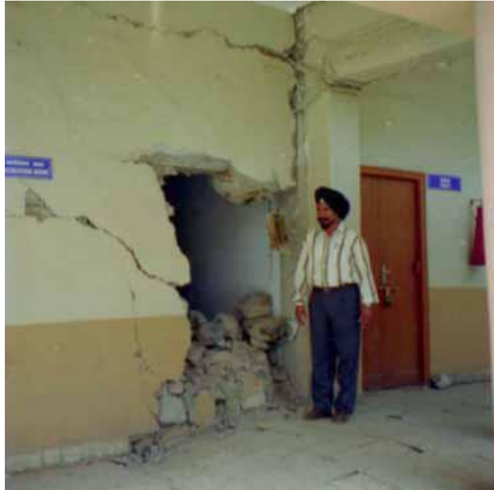
Fig. 1 Structural damage to a building caused by an earthquake[4]
