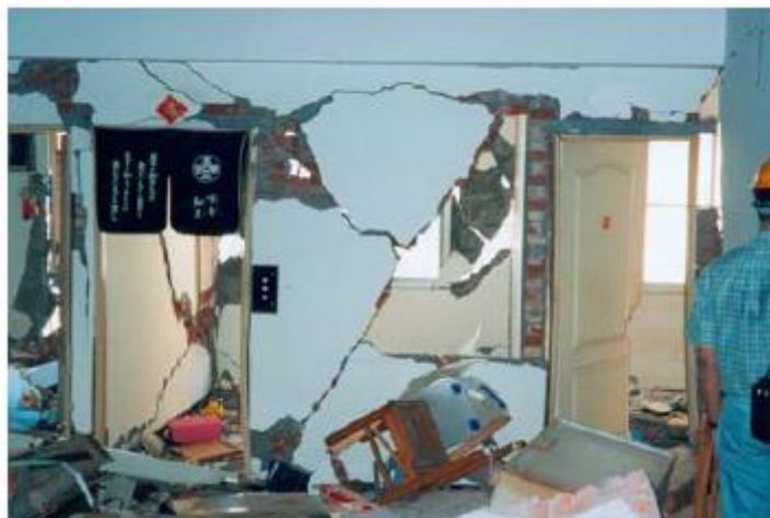
Fig. 2 The broken internal wall and the debris on the ground [5]
