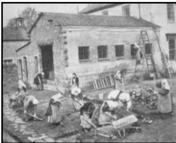
Figure 6.2 Carmelite nuns on the building site of the Church of Our Lady of Assumption of St Therese, 1954. Source: Menevia Diocesan Archive
