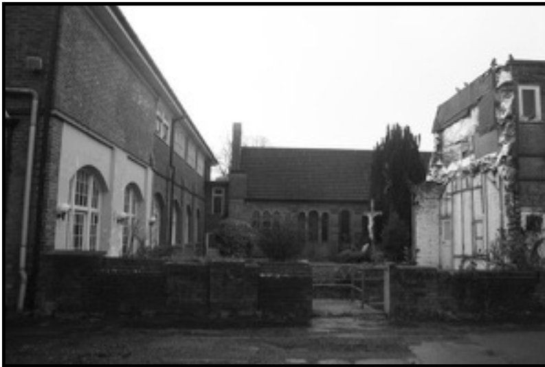
Figure 4.10. View of the partially demolished walkway between the penitents quarters and the penitents nave in the Church of the Sacred Heart, Waterlooville. Source: author.
