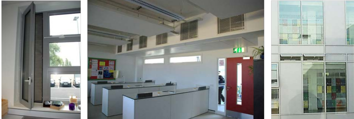
Figure 3: Cross ventilation strategy in Building 1 – operable windows (left), plenum air intake (middle) and the motorised vents on the corridor side (right).
