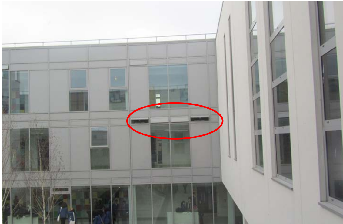
Figure 7: A number of motorised vents stuck open in winter in Building A which compromised the operation of the heating system.
