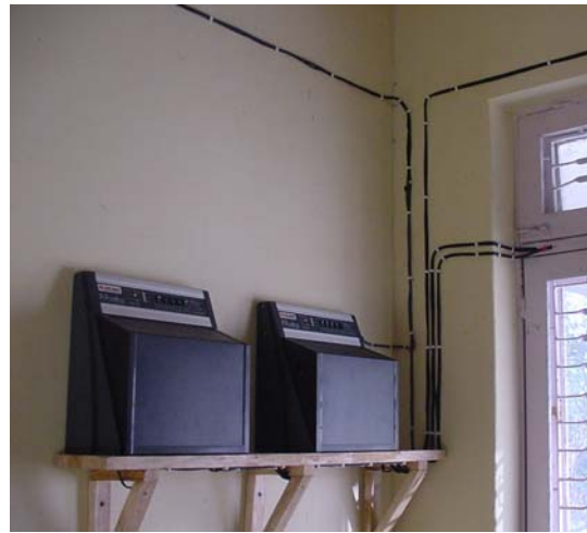
Fig. 3: Two of the battery charge controllers installed at Sankhe health post (NW room).
