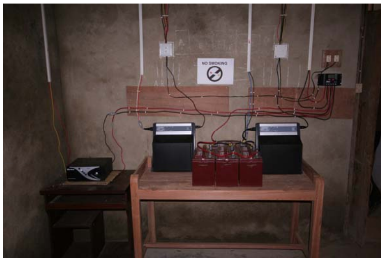
Fig. 8: Battery room showing the completed installation. The inverter can be seen on the far left, which is connected to the 4 batteries in the centre of the picture which power the PC and laptop. The charge controller for this system is mounted on the wall. The two black boxes contain the charge controllers and batteries for the two lighting systems (#1 & #2).
