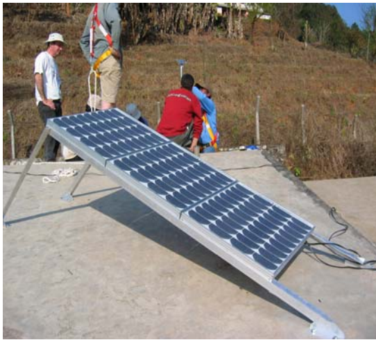
Fig. 2: PV array installed on Sankhe health post (SE side of roof).
