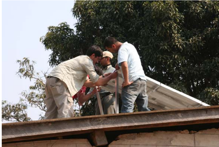
Fig. 7: Installation of the main array which was used to power the computers.
