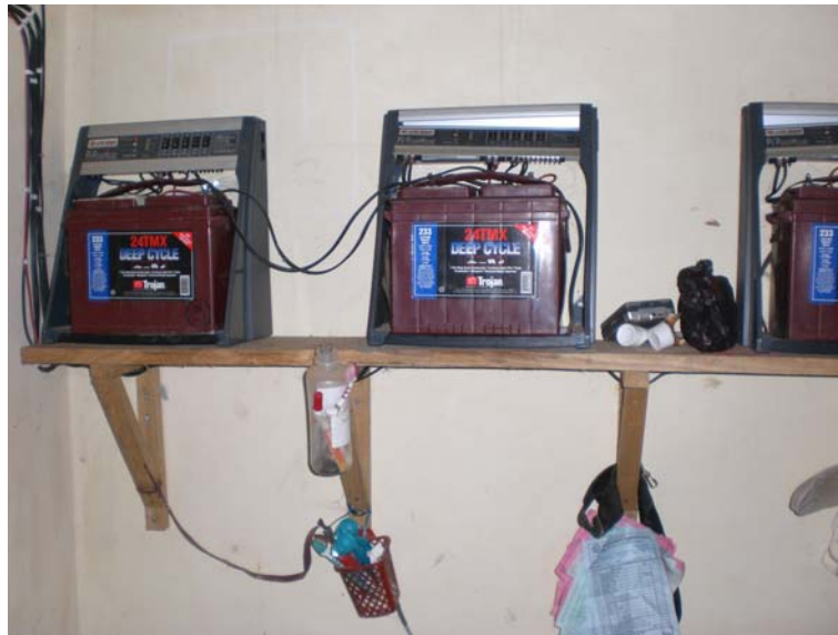
Fig. 6: Batteries located in the SW room of Sankhe health post (Feb. 2008)
