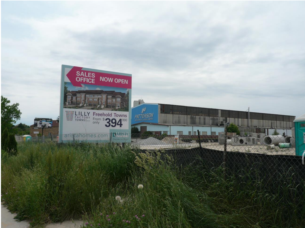
FIGURE 4: In inner suburban Scarborough, the former Lily Cup factory once produced disposable cups for fast food chains like McDonalds and Tim Hortons. And for a fleeting time, before it was demolished in 2010 to make way for the Lilly Factory Towns (now under construction), it was home to a South Asian banquet hall, and then a gathering place and Mandir (temple) for Bangladeshi Hindus. Part of a wider redevelopment boom in the area, the redevelopment of the Lily Cup and much of the industrial land around it brings new, more compact housing to the postwar suburb, but it ironically makes it less mixed use. Factories that once provided middle-income employment for area residents have been replaced by townhouses, while little new retail or office space has been added to the area. The final users of the old factory have in the meantime relocated to a small industrial building in nearby East York, having made temporary use of a nearby Royal Canadian Legion Hall for pujas and other special events in the interim (photo by Robert S. Fiedler).
