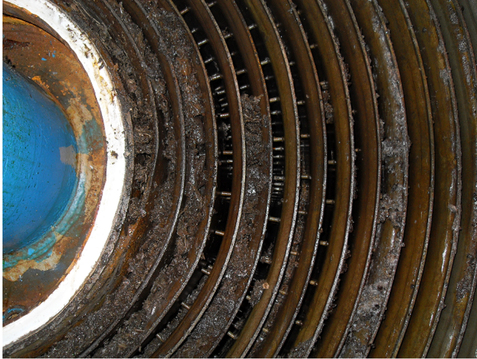
Figure 2: Photo of the spiral heat exchange from Huntsman Pigments's plant showing the carbonaceous build up on the equipment caused by the soya oil. The heat exchanger reduces the temperature of the pure \text{TiCl}_4 and the sticky carbonaceous build up reduces the efficiency. This build up is caused by impurities. Reducing these impurities therefore reduces downtime. For scale this heat exchange has a diameter of 2.5 metres
