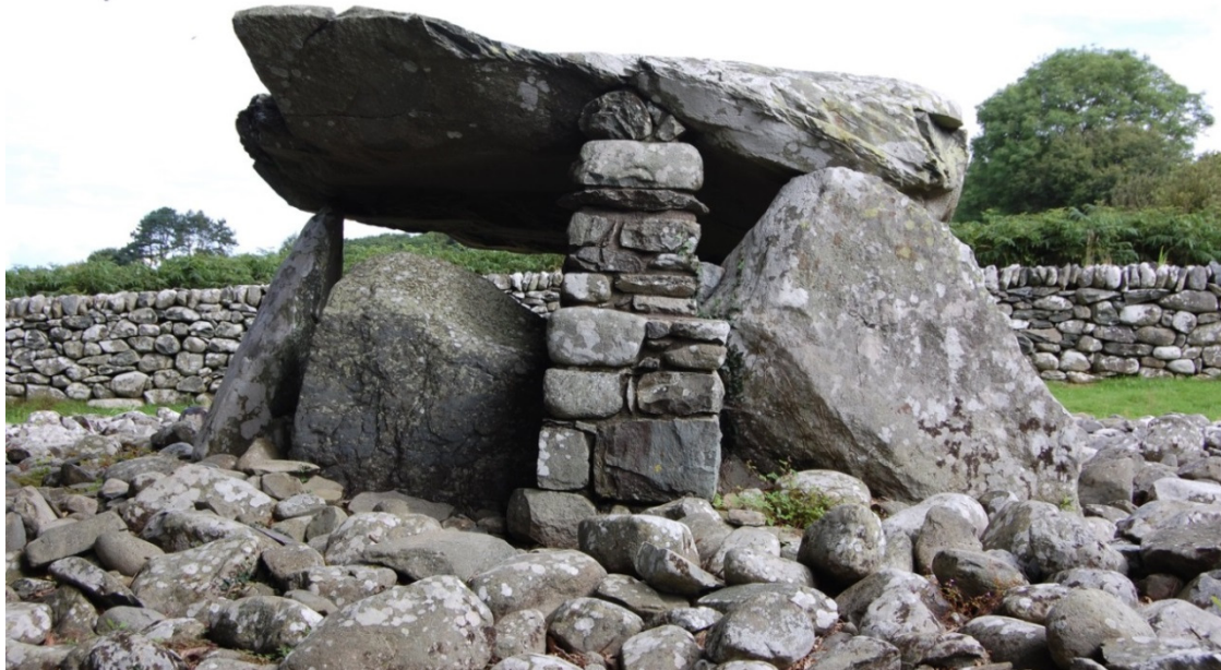
Figure 7.4. Stone pillar built as part of the conservation of Dyffryn Ardudwy chambered tomb
