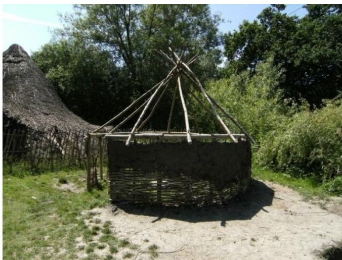
Figure 15 The construction activities area at the Peat Moors Centre showing the erected rafters and the pupils' daubing efforts.
