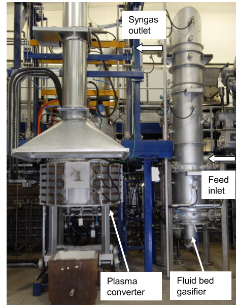
Fig. 2. APP demonstration plant, Swindon, UK.
