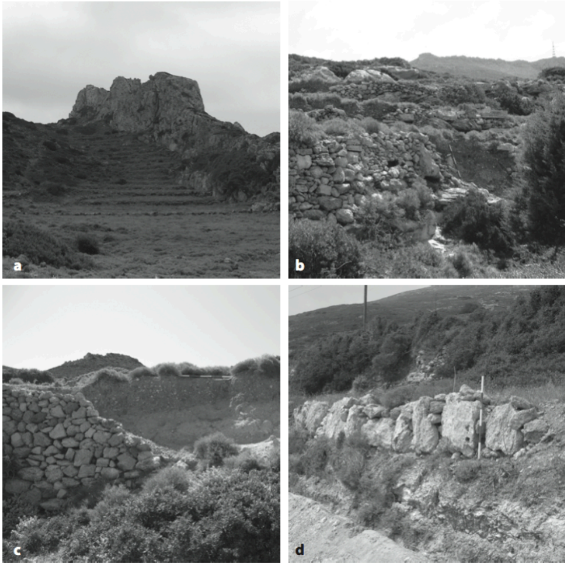
Figure 4. Terrace types and riser construction techniques: a) low cross-channel terraces in a tectonic valley on hard Cretaceous limestone, b) higher hillslope terraces collapsing on Neogene marl limestone (the Ch1 section is by the ranging pole in the foreground), c) a collapsed riser from a deep cross-channel terrace made entirely of even-sized Neogene limestone cobbles with at least two buried soil horizons behind it, and d) a riser from a hillslope terrace made of a basal course of large Neogene limestone slabs filled with smaller stones (the BO1 section is just out of view to the right).
