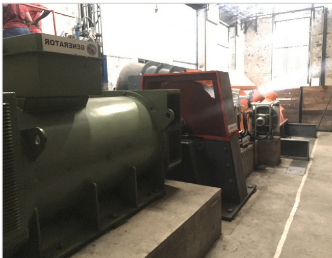
Fig. 7. Powerhouse structure with generation machinery at Zengamina hydropower station. Source: (Mbazima, 2024).
