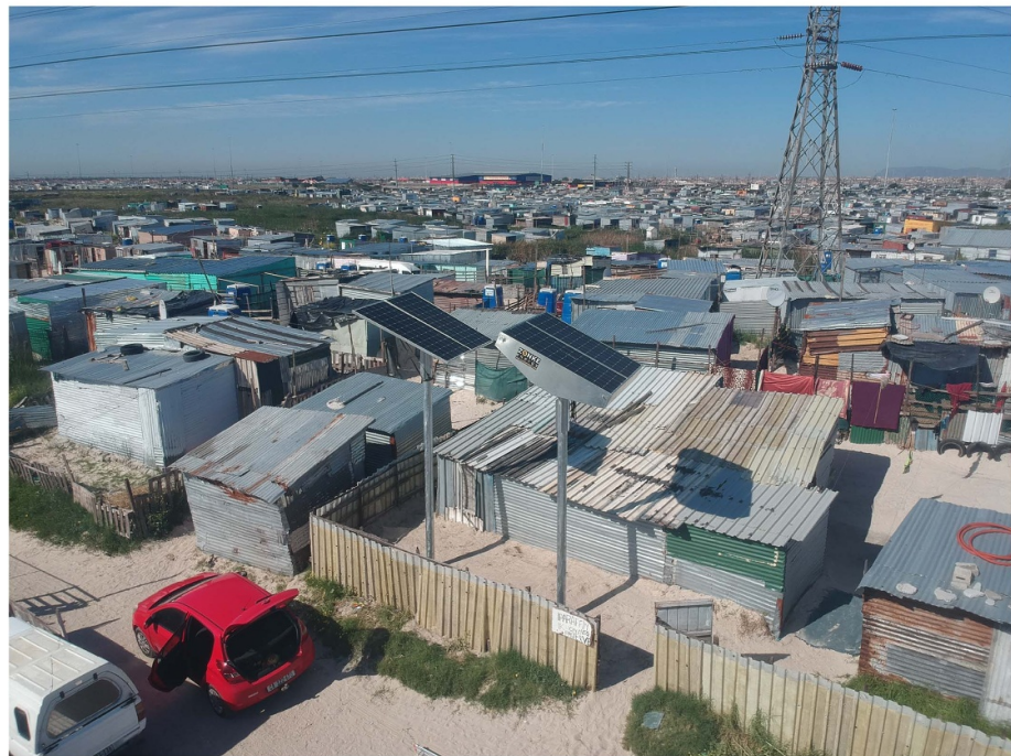
Figure 2. Some of the solar microgrids installed in the settlement (Photos: Authors).
