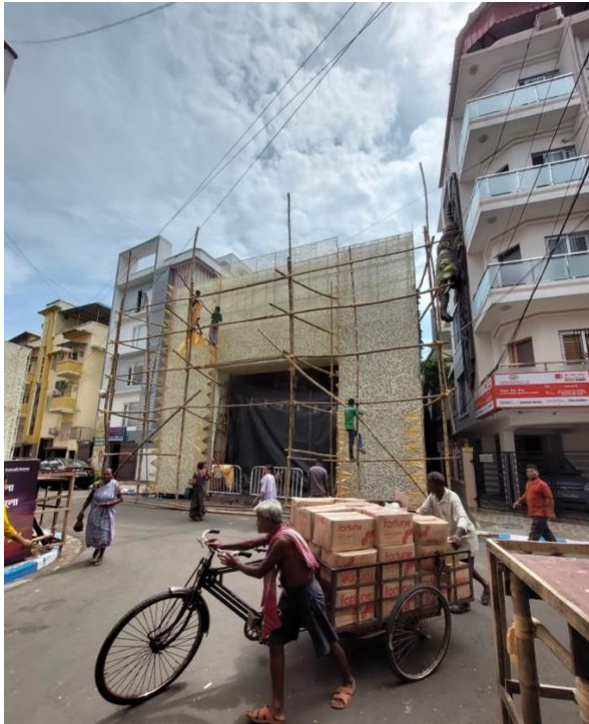
Mudiali pandal facade being constructed and the labors involved (2022). Note also the cart and cart-pullers in the foreground, delivering mustard oil, used for both cooking and ritual purposes. Photo: Subhrojyoti Mukherjee. Copyright: Swati Chattopadhyay
