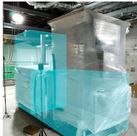
Figure 3: site logistics and equipment delivery use case. Pre-installation validation using BIM-AR shows the wrong orientation of the equipment compared to its orientation in the design model. Image courtesy of XYZ Reality Limited. (XYZ Reality, 2022)
