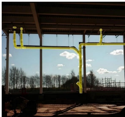
Figure 6 post-installation progress tracking using BIM-AR. Location deviations between installed rainwater pipes and their corresponding elements in the construction model. Image courtesy of XYZ Reality Limited (XYZ Reality, 2022)
