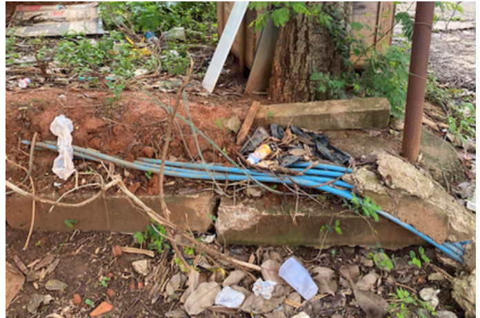
Figure 3: Collective water connection pipes prone to leakage and contamination.
