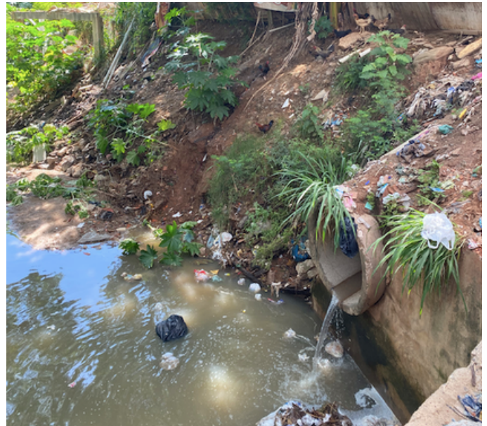
Figure 2: Local stream contaminated with liquid and solid waste.
