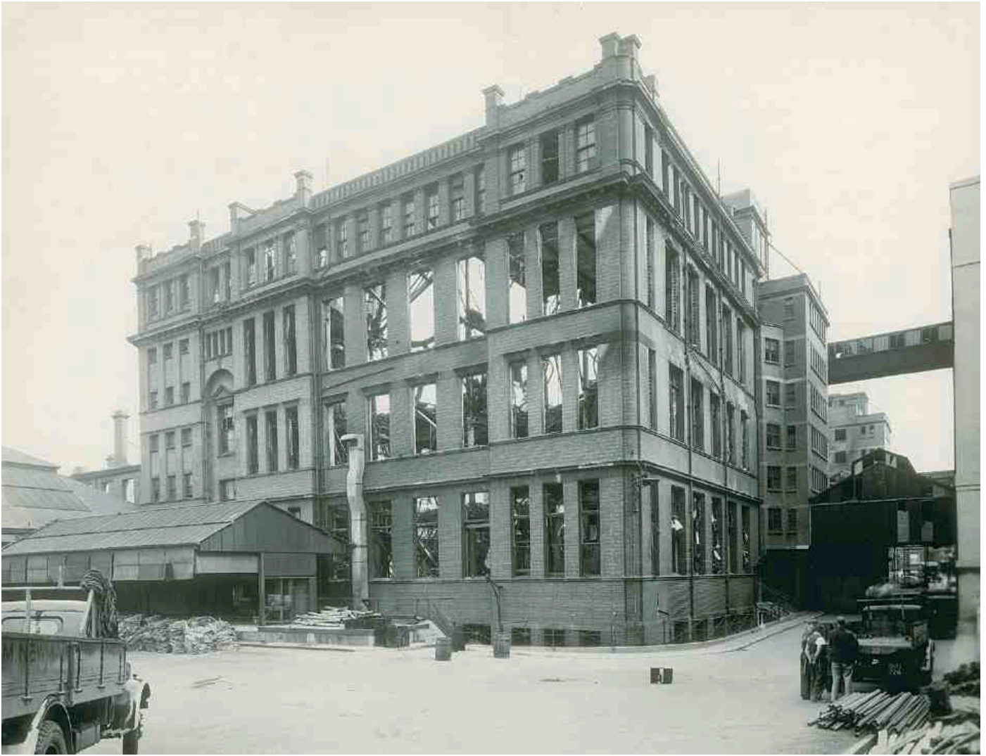
42. Parcel Office, south-west corner, following bomb damage, July 1943, showing steel-framed lavatory wing (right); highlevel walkway to letter office beyond
