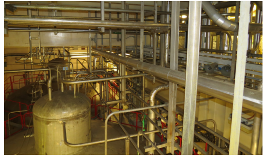
Fig. 2. Photo of a post-operational site including tanks with pipework to be dismantled at Sellafield [23].
