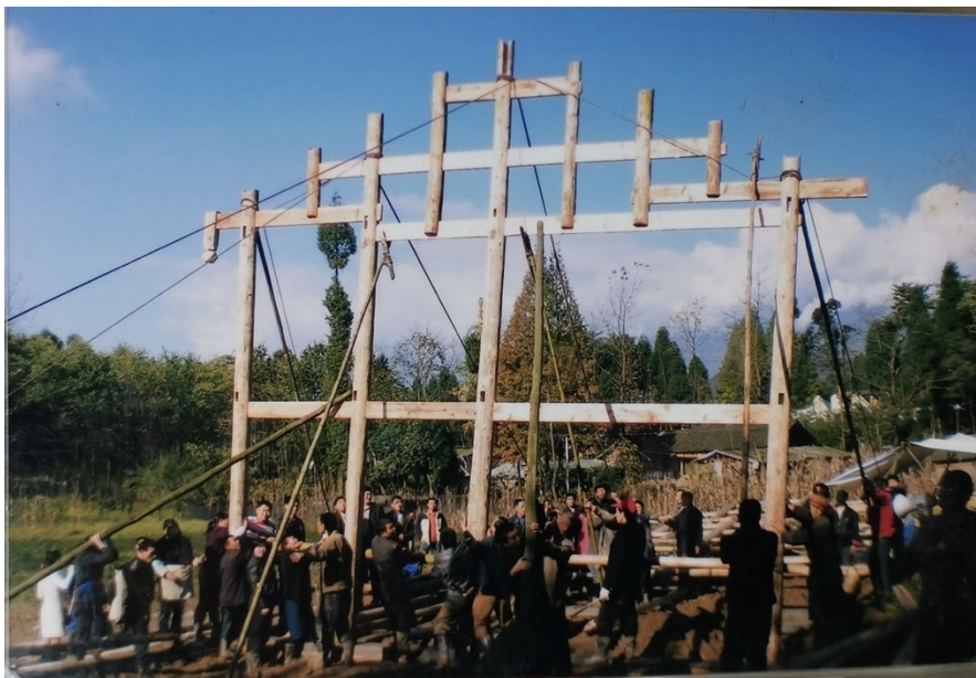
Figure 5. The Truss Made up of Columns and Beams (source: Daping Village Committee 2009).
