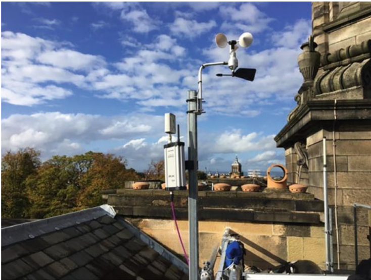
Fig. 8 Xirium Pro receiver installed on the roof of Modern Two (Photo: Brian Castriota)
