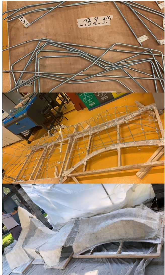
Figure 7. In-situ reinforcement system built with robotic rod bending, and the final prototype.
