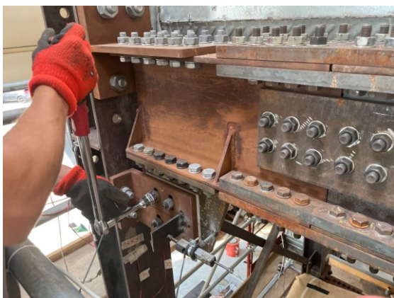
Figure 6 FDs bolts' loosening process for the BCJs.
