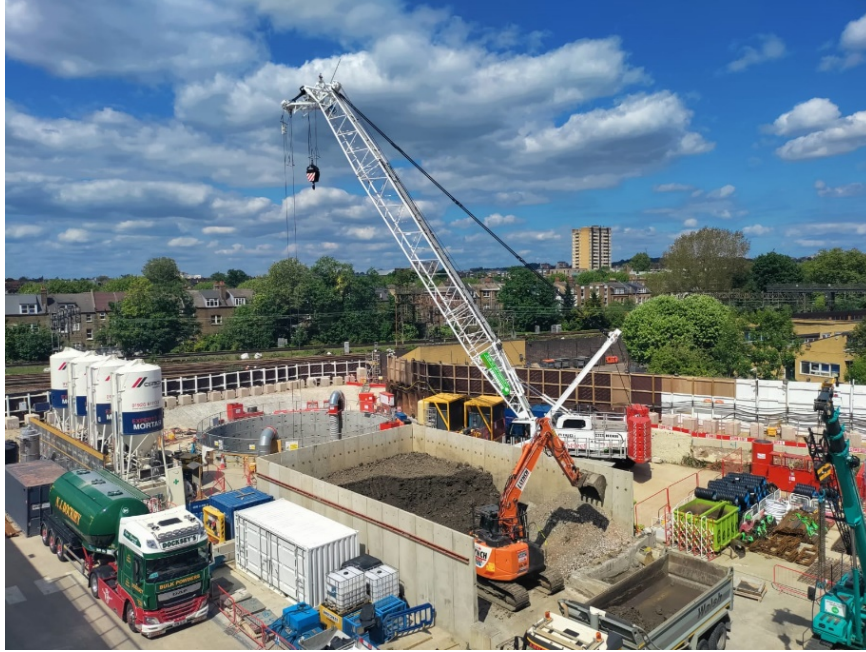
Fig. 1. A High Speed 2 construction site for a concrete shaft and collected excavated London Clay.
