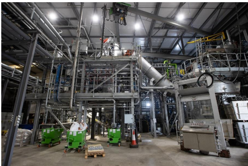
Figure 6: Gasifier at ABSL Swindon plant
