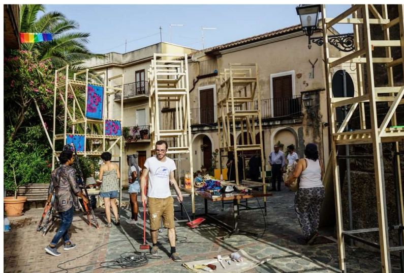
Figure 3. Construction of mobile shelving towers in 2018 (Source: photograph by Silvia Gin and Zeshan Mazhar)
