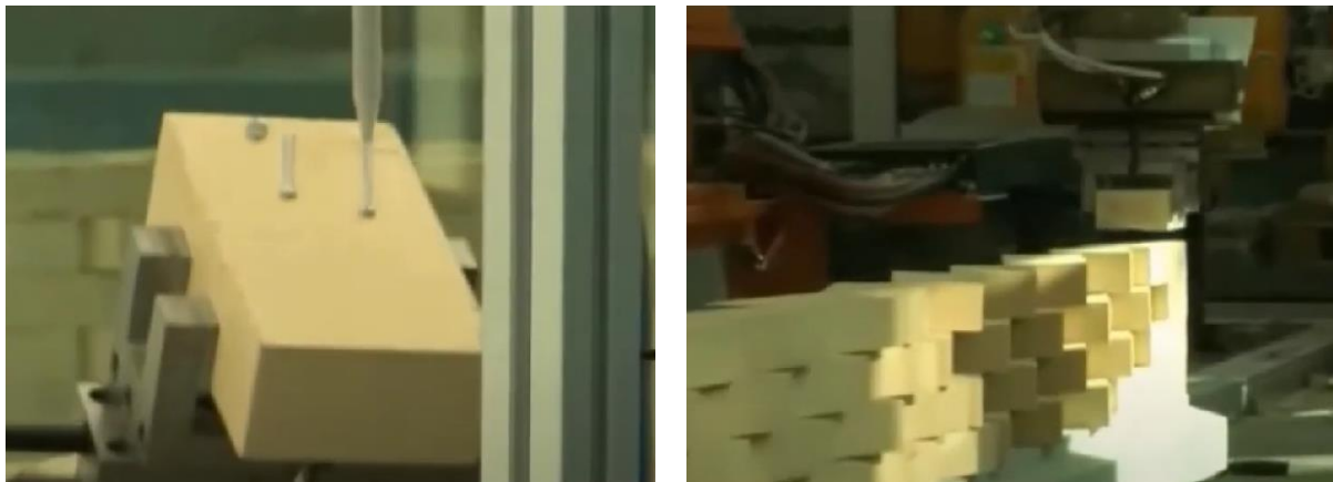
Figure 12: Bricklaying as reinterpreted by automation, the construction of the Gatenbein winery brick modular panels, © MuDA ( https://www.youtube.com/watch?v=FhL-hWPpnzA )
