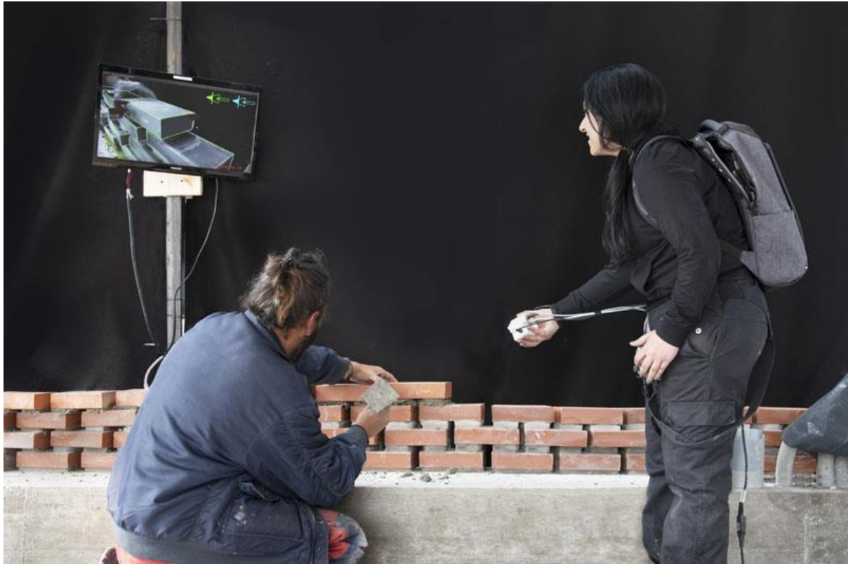
Figure 10: Bricklayer and assistant's hands at work on the Kitrvs winery brick skin, © Gramazio & Kohler ( https://gramaziokohler.arch.ethz.ch/web/e/projekte/371.html )
