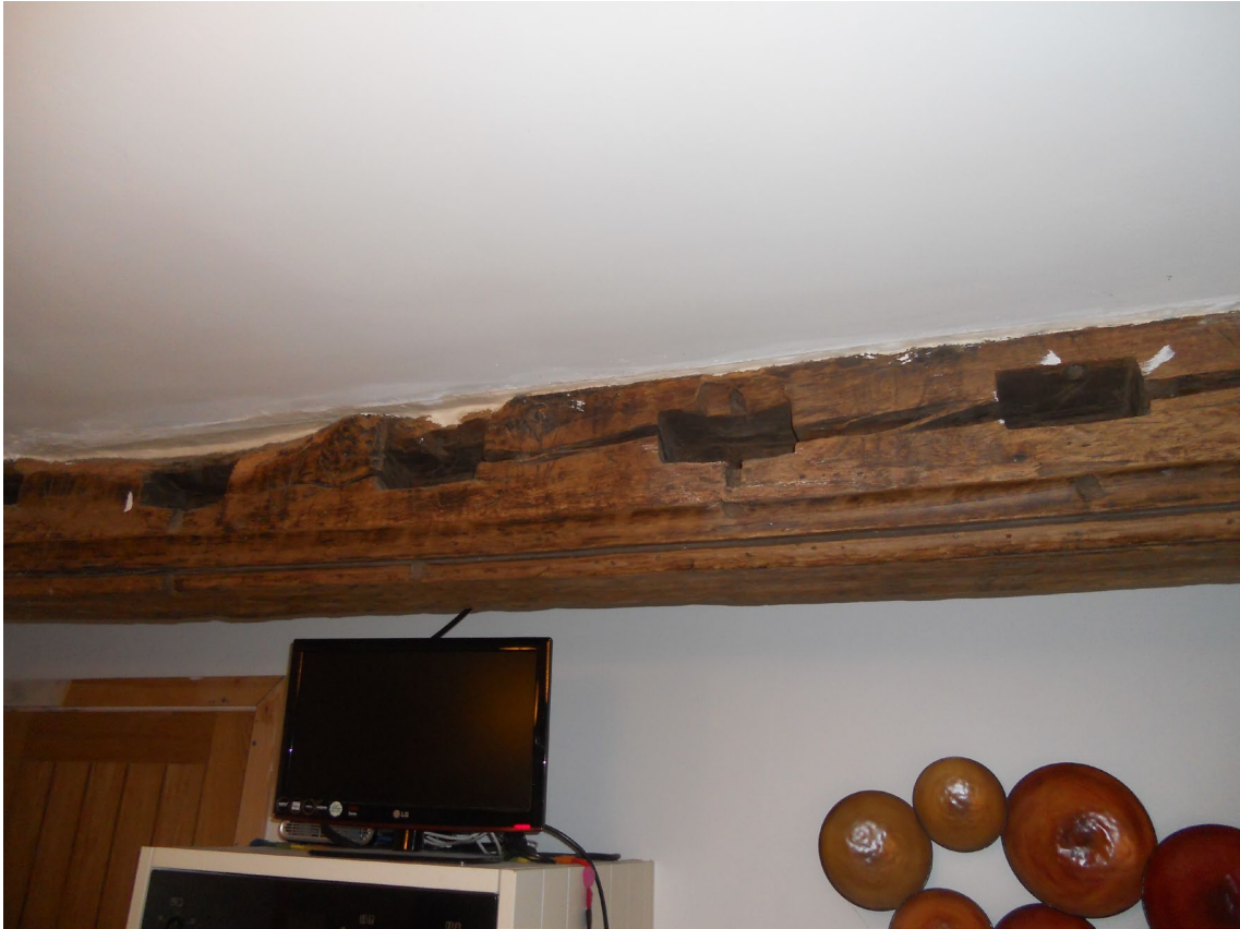
Figure 6: View of the cavetto and ogee moulded beam in 1A Market Place (photograph Martin Bridge)
