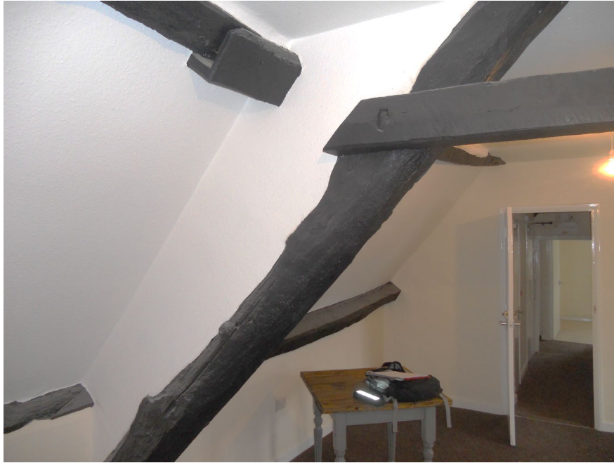
Figure 4: View of Truss B, the elm replacement truss, which was not sampled for dendrochronology (photograph Martin Bridge)
