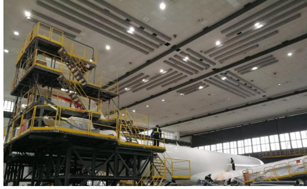
Fig. 2c The photograph of air supply module in ventilation system
