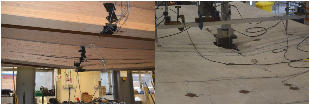
Figure 11 – Primary failure modes of (a) specimen S1 (joist fracture), and (b) specimen S2 (concrete punching)
