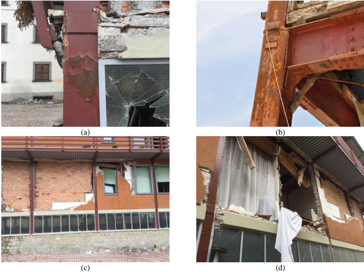
Figure 1. Typical damage on existing steel MRFs: (a) yielding of structural components; (b) fracture (ultimate failure) of structural components (from Ricles et al. , 2011 [35]); (c) cracking of masonry infills; (d) collapse (out-of-plane failure) of masonry infills.
