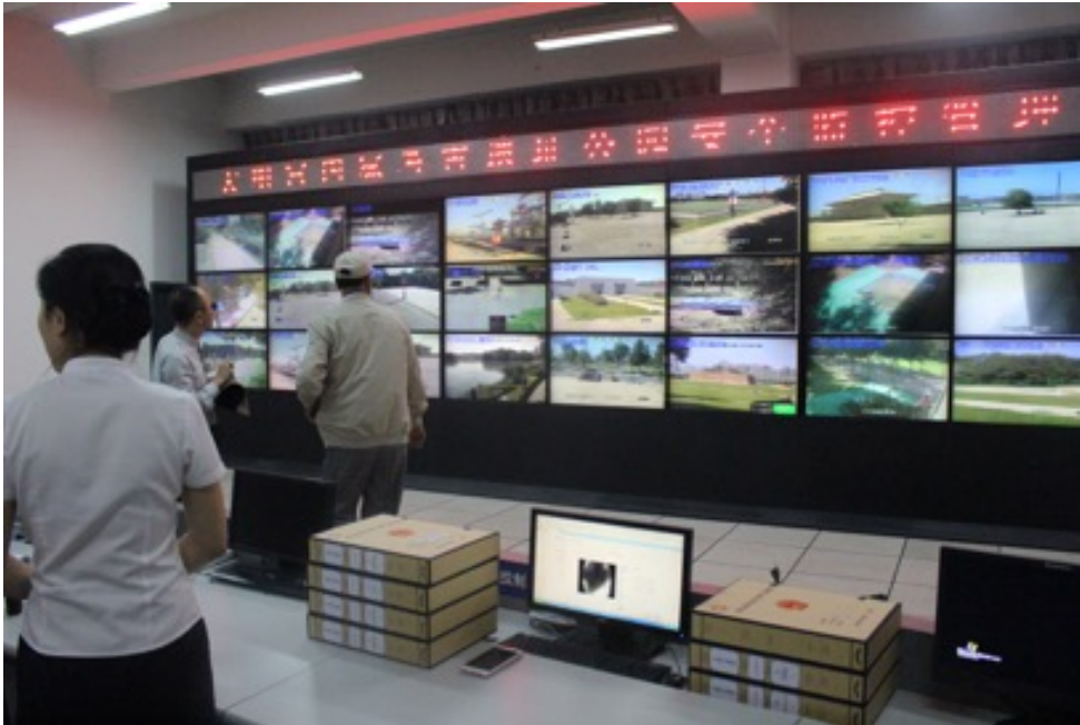
Figure 13 The control room of the protection unit
