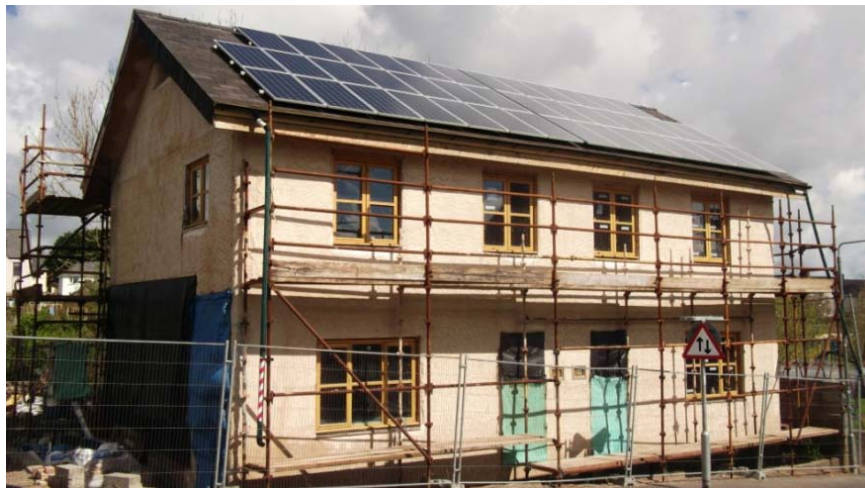
Figure 6: Pembroke Dock strawbale houses – view of south elevation awaiting final render coat
