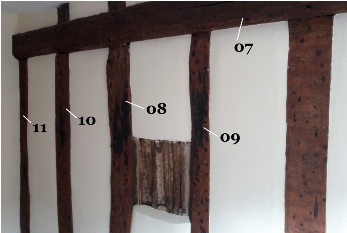
Figure 6: Gable wall of the St Austin's Lane building showing an abundance of burn marks and the locations of some of the timbers sampled (photograph Martin Bridge)
