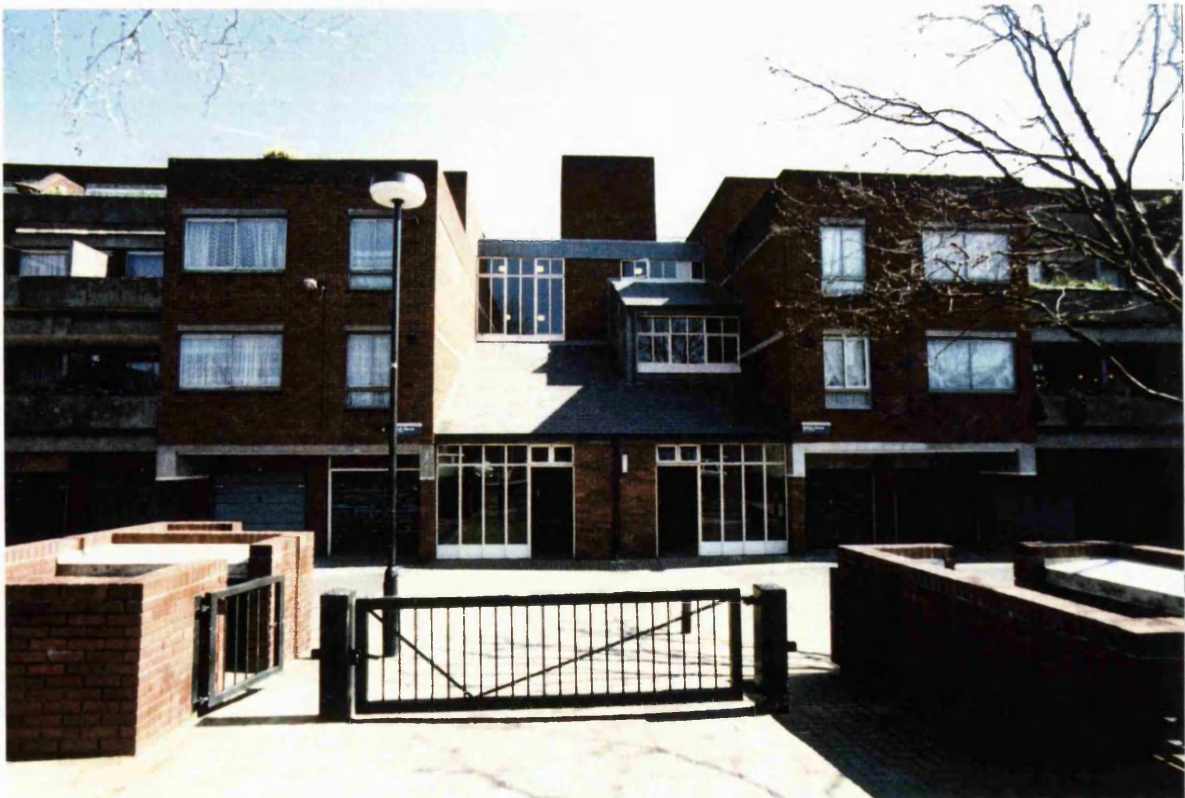
Plate 34: A new stairwell that has been created between blocks by filling in the gaps.
