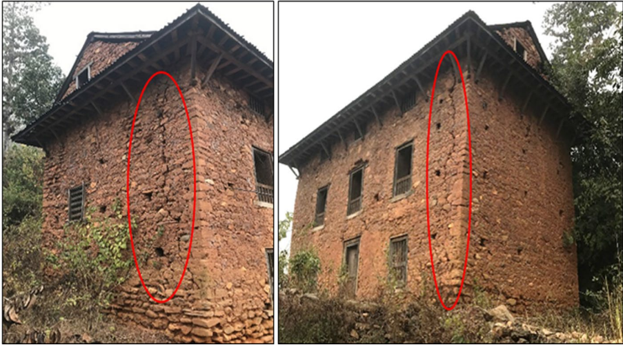
Fig. 19 Actual damage due to the 2015 earthquake in the case study PRE-SMM building from Sindhupalchowk district (vertical separation cracks have a maximum width of about 20 mm)
