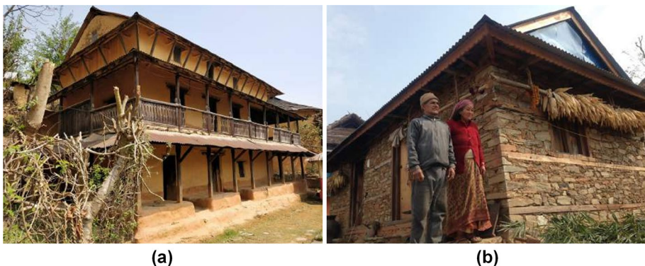
Fig. 6 SMM houses with seismic resistant features of timber elements: a an 80 years old PRE-SMM house in Syangja district that has survived three major earthquakes including the recent 2015 Gorkha earthquake and b a newly built POST-SMM house (HRRP 2018) (Images reproduced with kind permission of HRRP Nepal)
