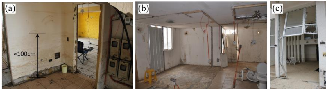
Fig. 5 – (a) Run-up marks left on the walls; (b) non-structural elements washed away in first story housing units; and (c) non-structural damage in first story common areas
