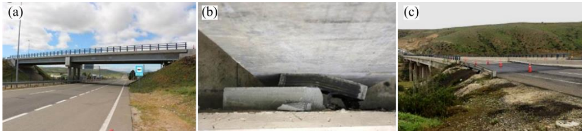
Fig. 9 – (a) Talinay underpass; (b) creeping and 16 cm residual displacement of the elastomeric bearings on the superstructure of Talinay underpass; and (c) temporary asphalt ramp on the south access of Teniente Bridge
