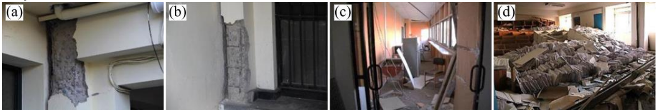
Fig. 3 – (a, b) Concrete spalling at Illapel hospital; (c) non-structural damage at Coquimbo hospital; and (d) shelves collapse with medical records at Coquimbo hospital
