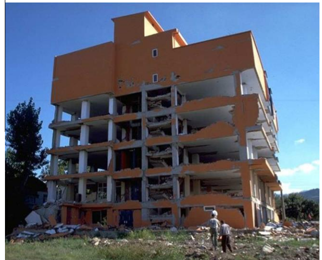
Fig. 5. A photograph of a façade of the Kocaeli residential building [45].
