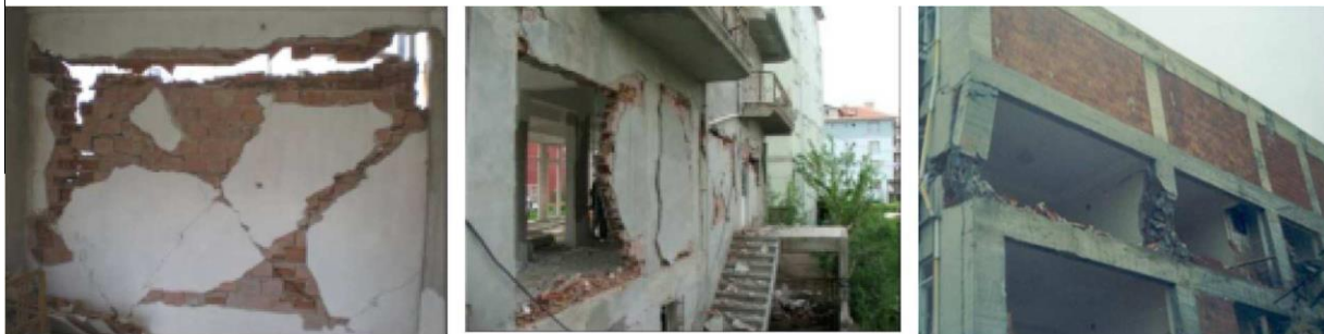
Fig. 3. Typical out-of-plane failure of URM infills in RC framed building, showing top-down collapse creating new voids that reveal the underside of the RC beams.
