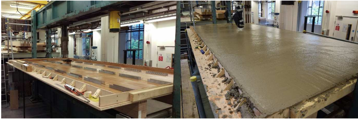
Figure 6 - Formwork for three-joint specimen (a) before concrete pour, and (b) following the concrete pour
