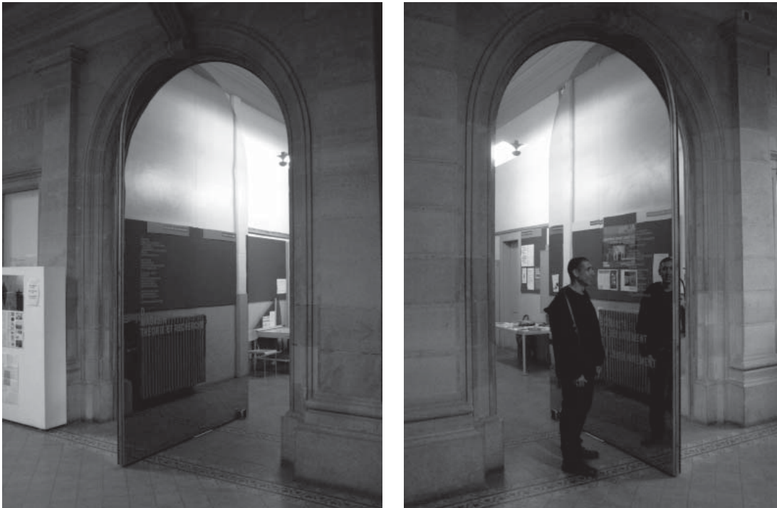
FIGURE 14: ‘INVISIBLE’ FIRE DOORS
