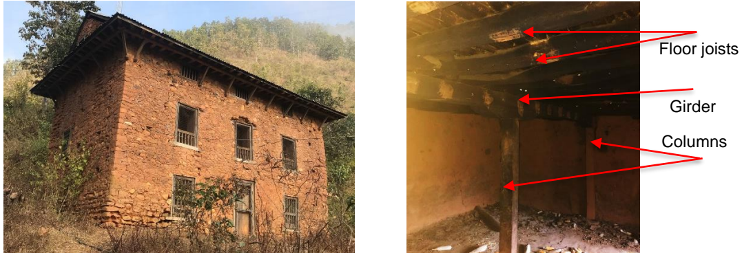
Figure 4. Photograph of a typical PRE- SMM building in Sindhupalchowk district (left) and timber framing structure (right).
