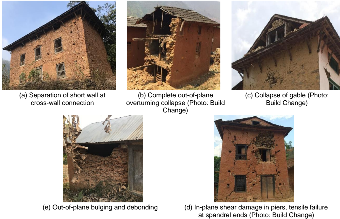
Figure 7. Main failure mechanisms of PRE-SMM typology observed in 2015 Nepal earthquake.
