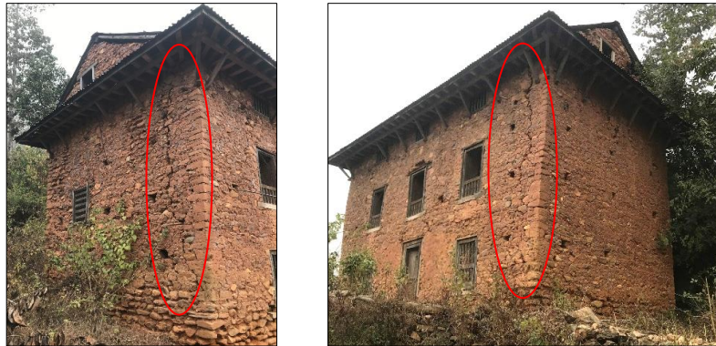
Figure 14. Actual damage due to the 2015 earthquake in the case study building from Sindhupalchowk district. Vertical separation cracks have a maximum width of about 25 mm.
