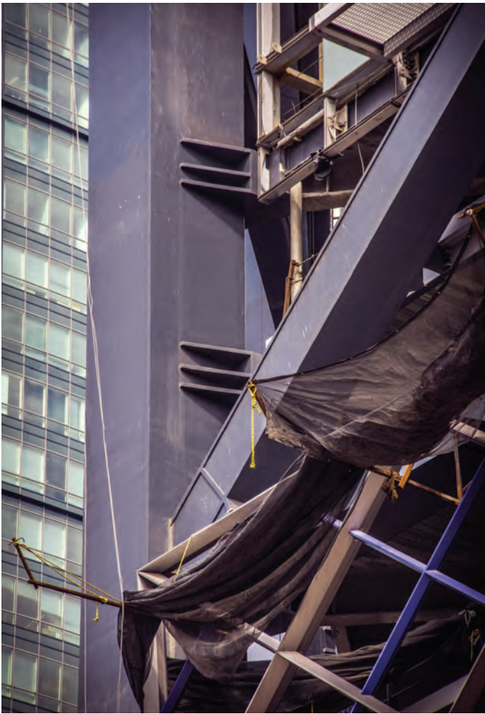
Figure 5. The “Crocodile Clamp” shown here during construction. The tectonic of the connection clearly express the flow of forces and “bites” into the main column. It is a legible part of the system. (Source: Rogers Stirk Harbour+Partners) 图5. 施工中展示的“鳄鱼夹”。连接处的构造清楚地表达出力量的流动性和主柱的“啮合”。这是系统清晰可辨的一部分。(来源: Rogers Stirk Harbour+Partners)
