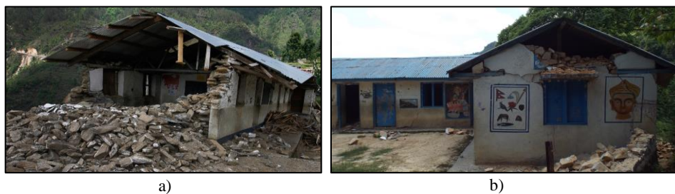
Figure 1. a) Heavily damaged dry rubble stone masonry school building and b) non-structural (gable) damage to a stone in mud mortar masonry school building in 2015 Nepal earthquake (Photo credit: The World Bank)
