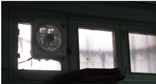
Figure 3. Small ventilation system with poor insulation
