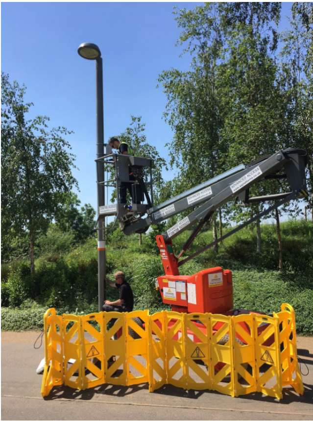
Figure 8: Typical installation of a Living Lab sensor
