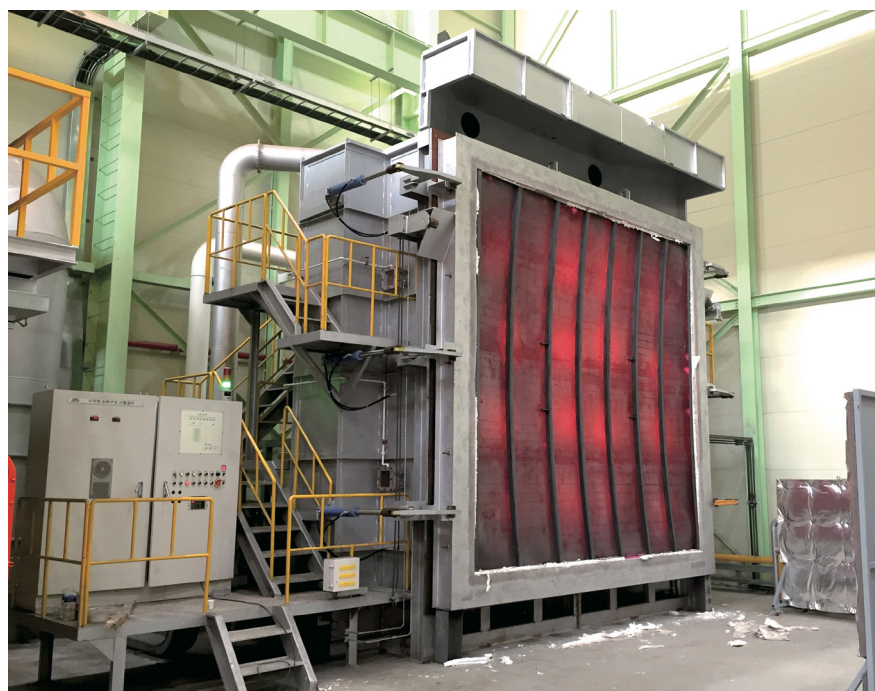
Figure 3. Vertical-type furnace test facility
