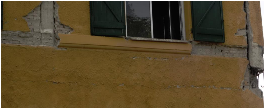
Figure 18. Damage to Non-Ductile Reinforced-Concrete Frame in Amatrice
