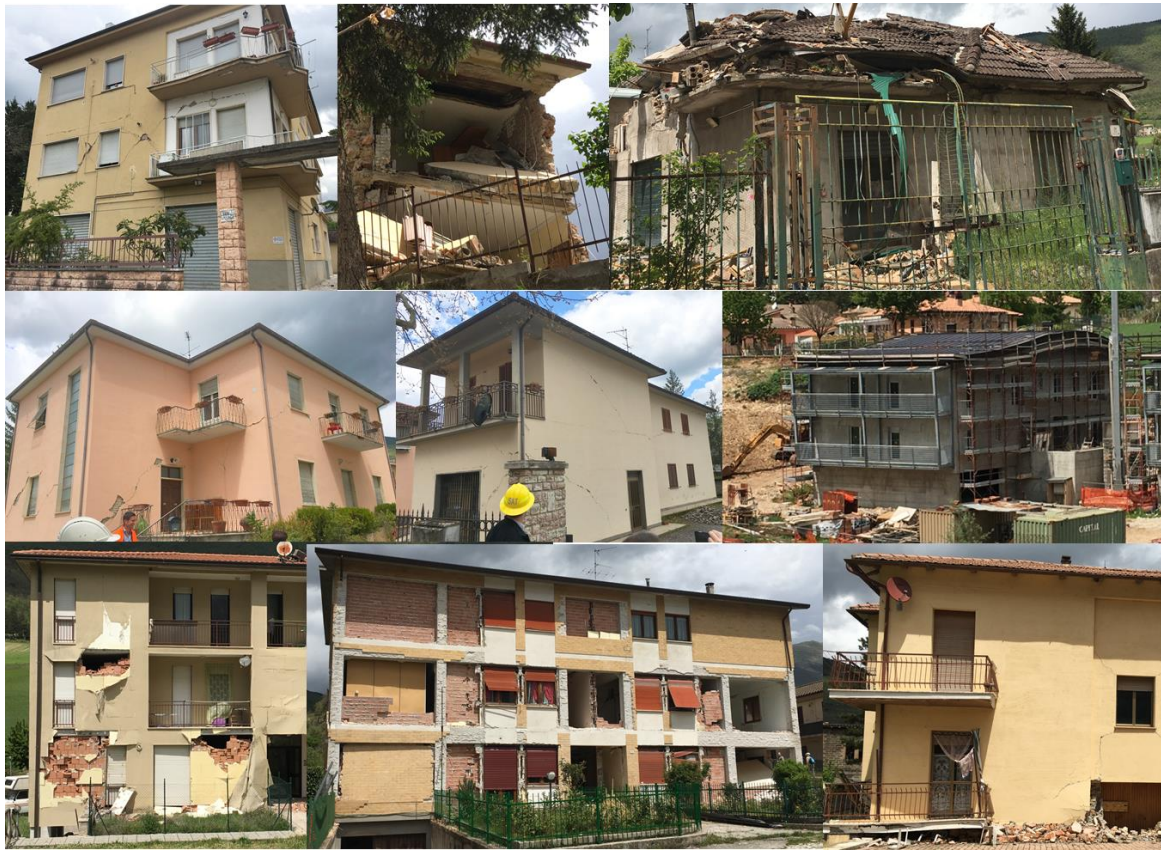
Figure 9. Representative Buildings and Damage in one area in the Periphery of Norcia, May 2017
