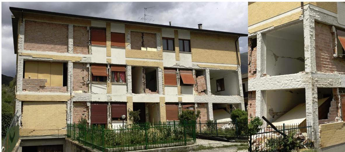
Figure 17. Representative Reinforced-Concrete Building in Norcia
