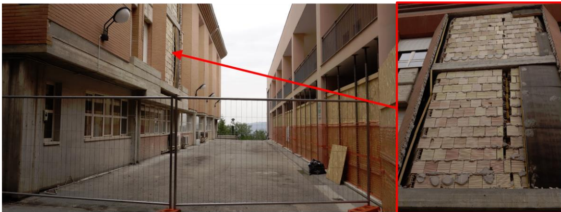
Figure 11. Hospital in Amandola after August 24th Earthquake
