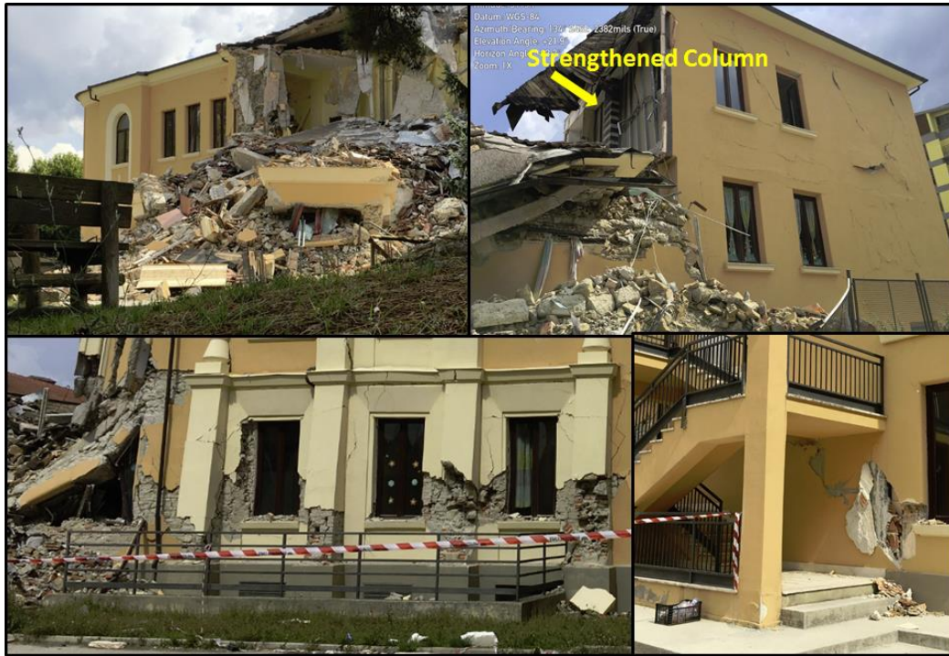
Figure 12. Primary-School Collapse in Amatrice, September 2016
